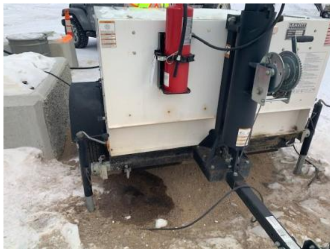
Dec 13, 2021 – Junction Camp, light generator leak, staining visible
