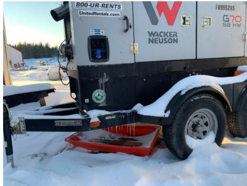
Spill tray under generator.
