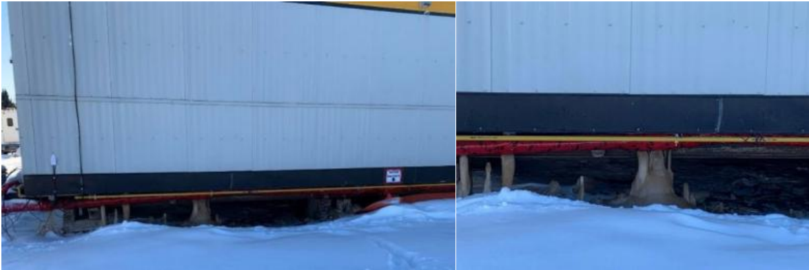
Photo 11: Pipestone Camp – Leaking pipe under rec trailer.
