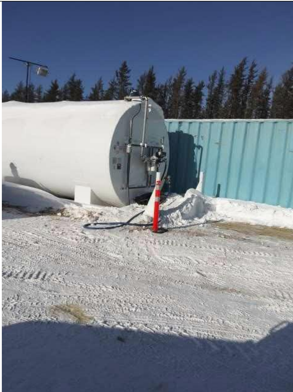
Figure 4: Potable water container not labeled
