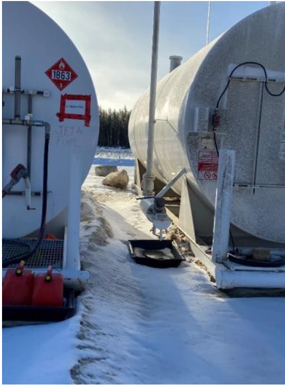
Above ground fuel tanks with signage and spill trays
