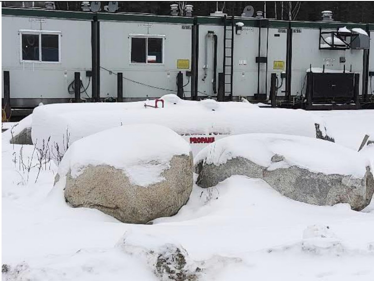
Figure 3: Bulk propane storage for camp heat
