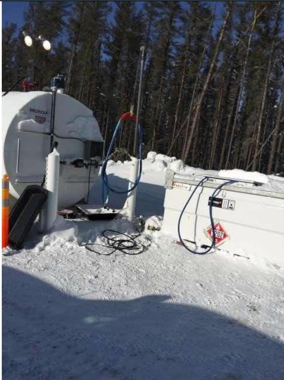
Figure 1: No vehicle barriers in place
