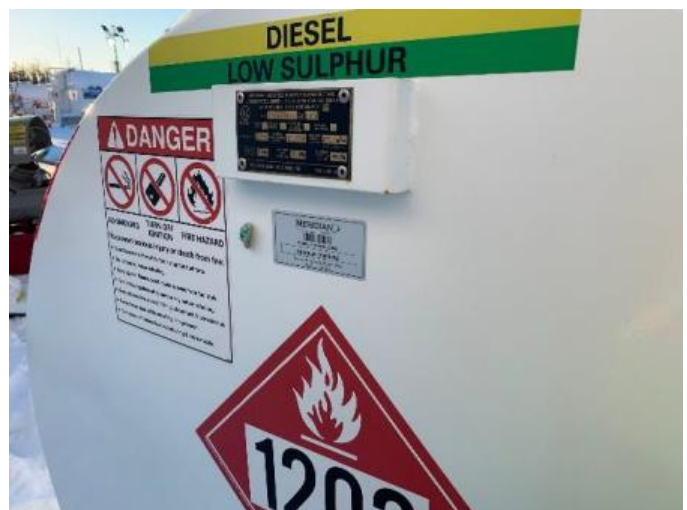
Fuel labels and plaque on tank in Pickle Lake yard.
